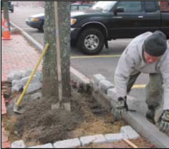
In the Millyard, tree wells are widened to ensure healthy growth and sustainability.
