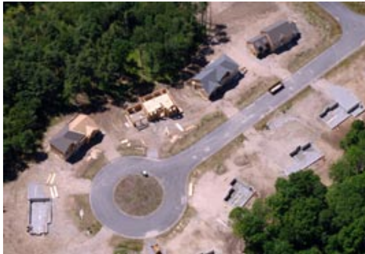
Large new homes are under construction near Manchester Airport. The city's rebirth is attracting new residents, many fleeing high taxes in Massachusetts.
